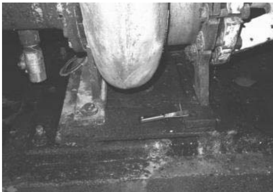
Figure 16-12 Misalignment can be detected via physical signs
