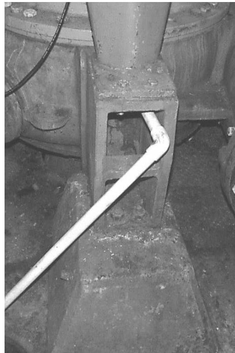
Figure 8-34 - Picture of one Pump Foot
