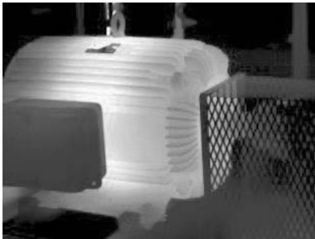
Figure B-10 A thermographic image of a motor
