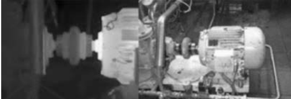
Figure A-21 Thermographic and photographic image of overheated bearing
