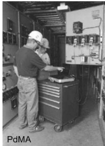
Figure A-37 Dynamic On-line Tests can be done at the electrical panel.
