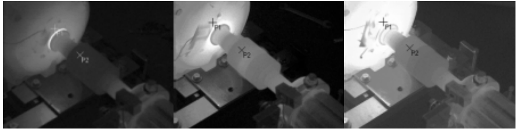
Figure 16-13 Thermal imaging showing heat buildup due to misalignment
