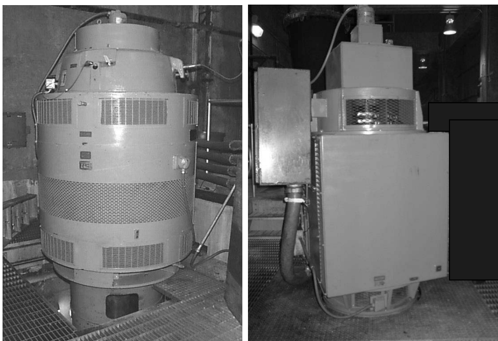
Figure 8-20 - Left – New Motor (pumps 1 & 2), Right – Old Motor (pumps 3 & 4)
