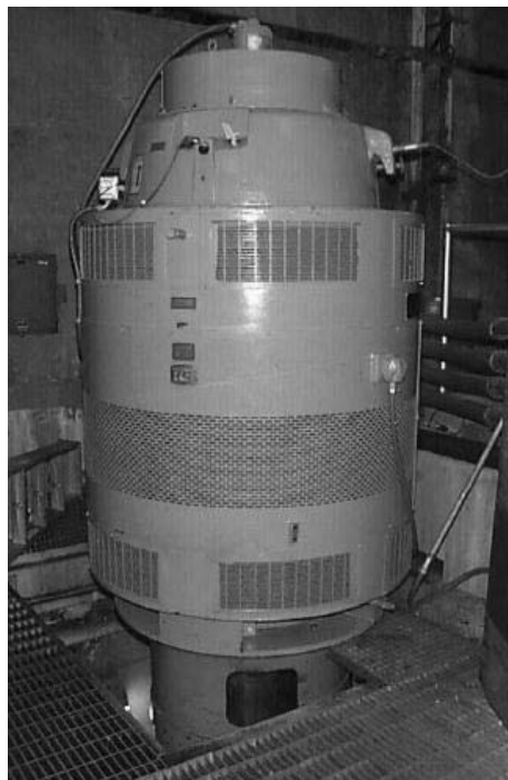
Figure 8-33 - 33 800 HP vertical pump used for ODS
