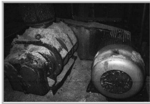
Figure 18-40 Belt drives and gear boxes produce multiple shaft running speeds
