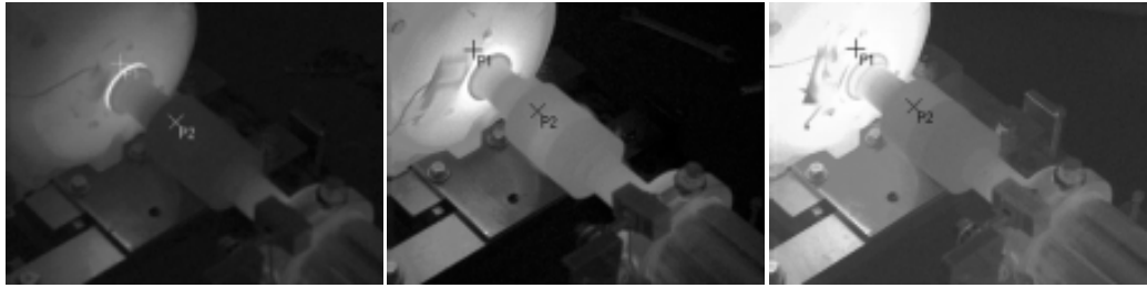
Figure 12-13 Thermal imaging showing heat buildup due to misalignment
