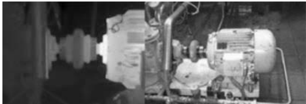
Figure 23-24 Thermographic and photographic image of overheated bearing
