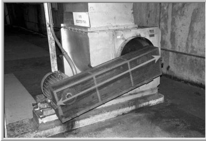
Figure 9-30 - Collect vibration measurements in-line with the belts.
