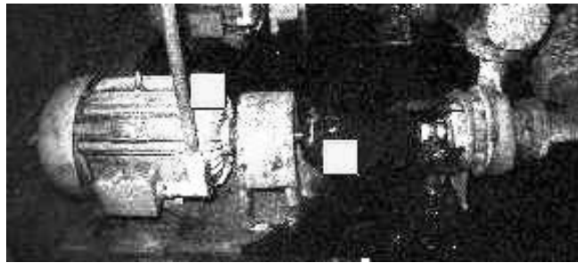
Figure 11-14 - Cooling Water Pump #2
