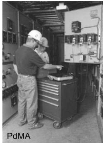
Figure 23-42 Dynamic On-line Tests can be done at the electrical panel.
